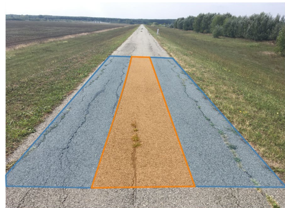
Fig. 2 Position of fissures on the paved dam crest
