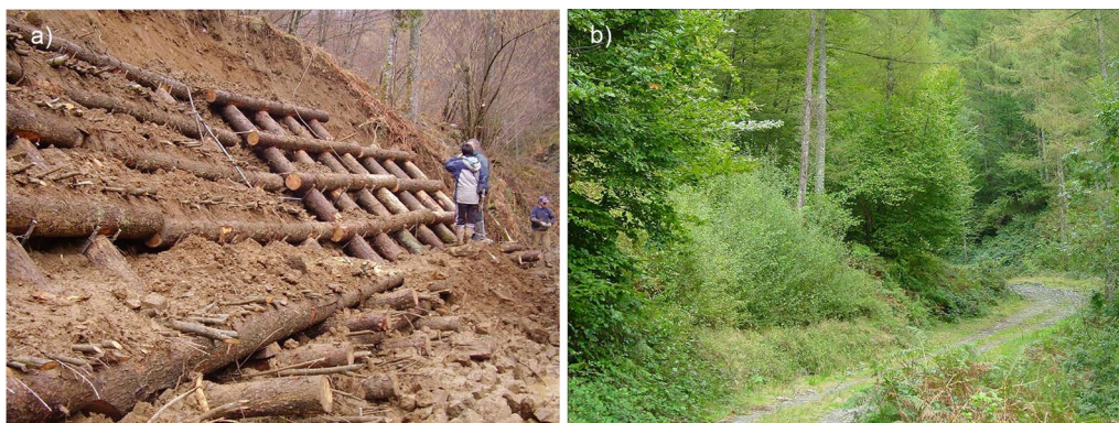
Fig. 8 Example of live crib walls along a mountain road in Leizaran, Spain a during construction and b after plants establishment. The wood structure is almost all covered by vegetation. (Pictures courtesy of P. Sangalli, European Federation of Soil and Water Bioengineering https://efib.org/ )
