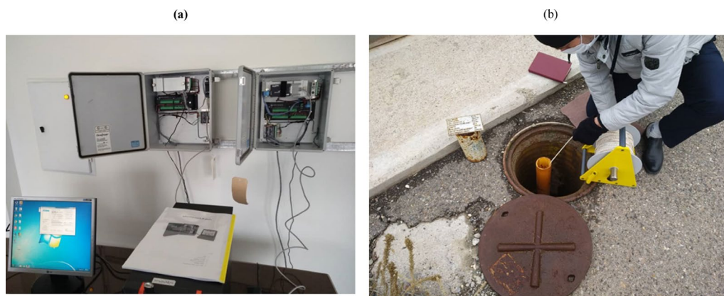
Fig. 4 Madani Dam: a Electronic equipment control room b Manual reading
