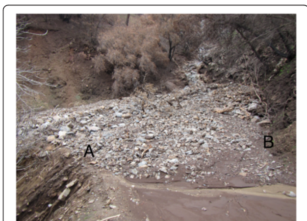
Figure 2 A photo showing one of five debris flow deposits blocking Lumsden Road, a native-surfaced Forest Service road accessing the Tuolumne River east of Groveland, California.
