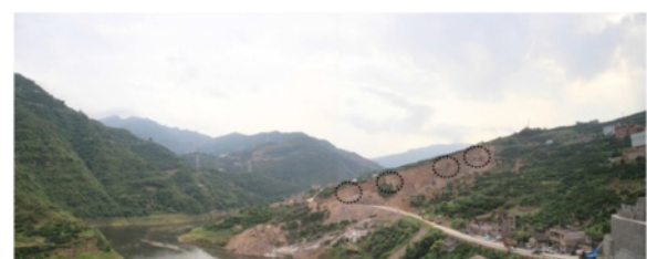
Fig. 13 Lateral view of the Shanshucaao Landslide (taken on Sep. 12, 2014). The cliff is the northern flank cliff of the landslide. Black dotted lines are damaged parts of the rock bridge (fresh exposures)
