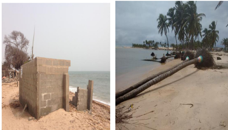
Fig. 3 Destruction at Fuveme and Ada due to increased erosion
